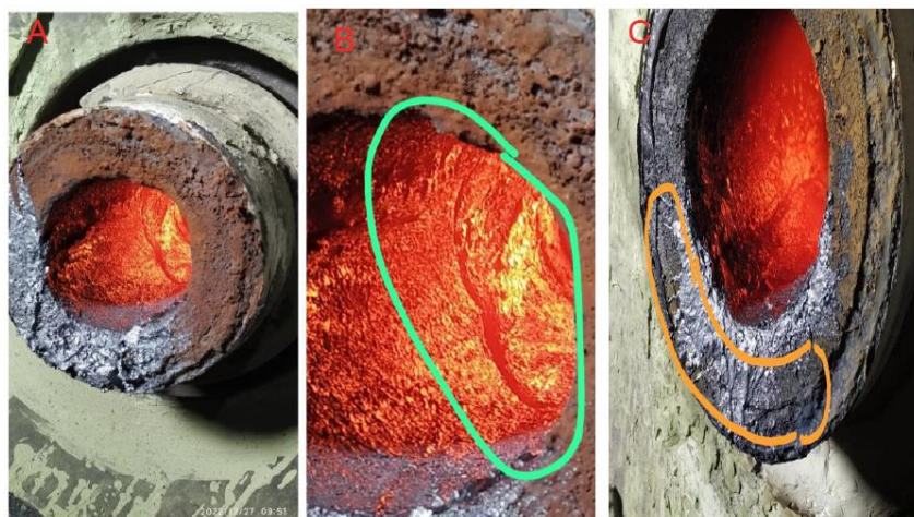
Fig. 1. Horizontal cracks & gauging in the conventional CNTs after 3 to 4 heats.
